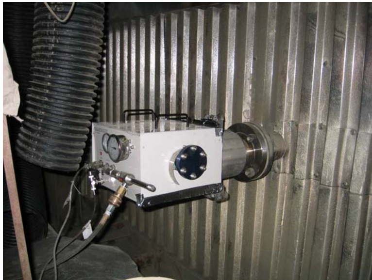
Figure 4. Detector Optics Enclosure Mounted on Power Plant Boiler
